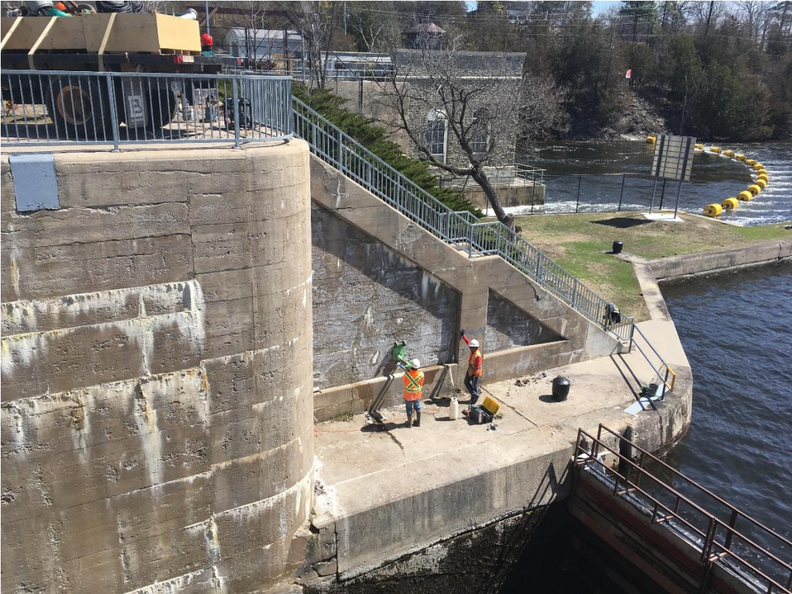
Workers conduct core sampling on the lock structure at Crowe Bay Lock 14 in April 2017
