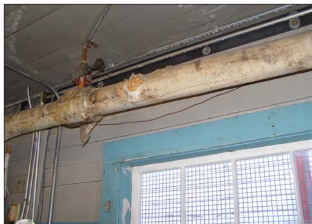
The mouldy insulation on this pipe was removed from Cannery Store office
