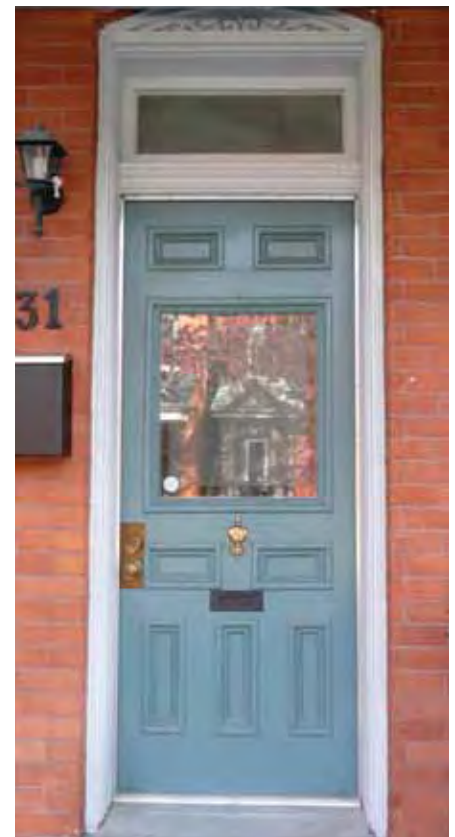
Doors are often targets for replacement because of security, energy efficiency or fire separation needs. Often it is possible to meet all these needs while retaining a historic door. Adding weather stripping can contribute greatly to a door's efficiency. Modern locks and locking mechanisms can often be installed with little damage. The fire rating of a solid wood door may meet certain code requirements.
