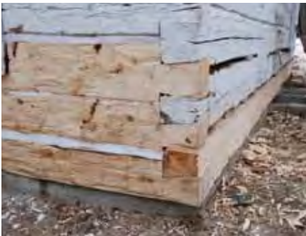
Deteriorated logs at the John Walter Historic Site in Edmonton were replaced in kind with hewn logs that used the originals as templates to reproduce tooling marks on visible surfaces. On close inspection, this distinguishes the new materials if the logs are separated in the future.
