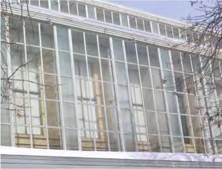
The character-defining transparency of the glass-enclosed factory wings of the National Printing Bureau in Gatineau, QC was preserved during conservation work on the glass and aluminium curtain walls. After the thin aluminium frames were cleaned, the opaque ribbed glass and clear plate glass were carefully reset in their original positions that reflect the pattern of solids and voids in the masonry wall behind.
