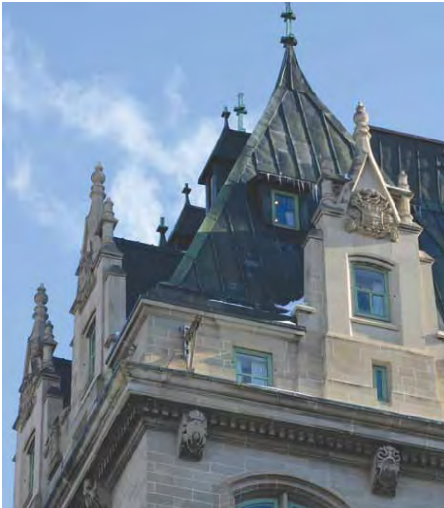
The steep copper roof of the Fort Garry Hotel in Winnipeg is defined by a multitude of small shed- and hip-roofed dormers, highly elaborate stone dormer facades at the corners, a wealth of pinnacles and large ornate chimneys.
