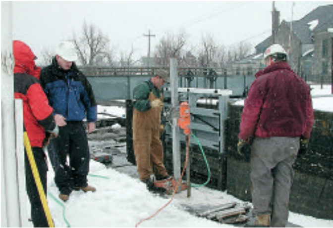
New techniques are now used for grouting, causing less damage to original fabric.
