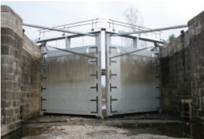
Originally made of oak, lock gates are now made of Douglas Fir due to the lack of oak of sufficient size.
