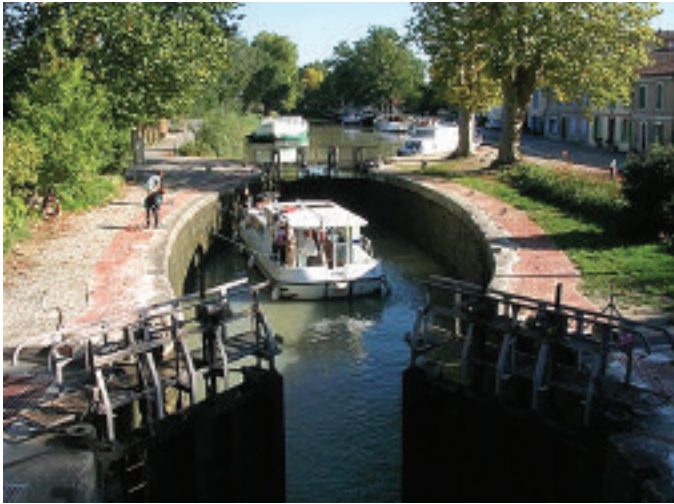
The Canal du Midi in Languedoc, France was designed with curved walls to resist the pressure of the earth and allow a larger number of boats into the lock.
