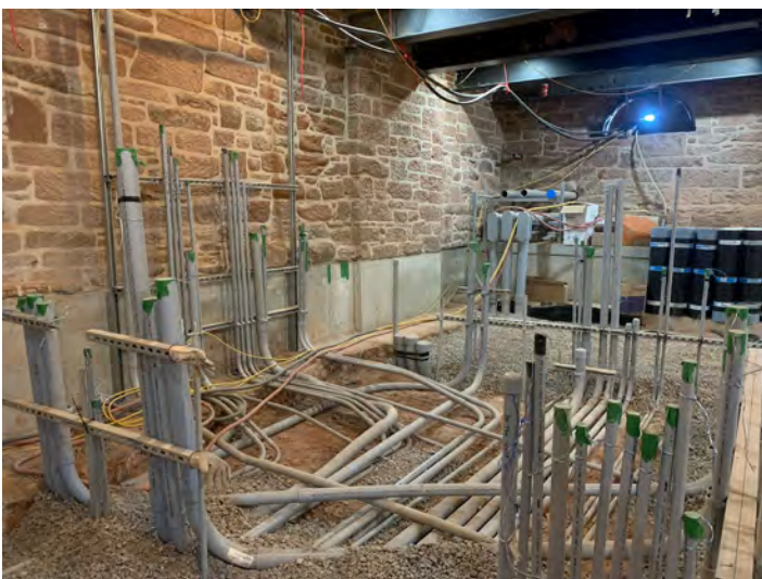
The basement floor under the slab is a maze of grey pipes for the underground services including septic, water, electrical, and communication conduits.
