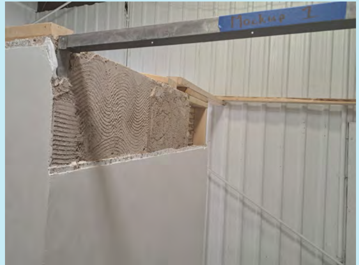
Mock-up of the lime plaster walls for Province House National Historic Site.
