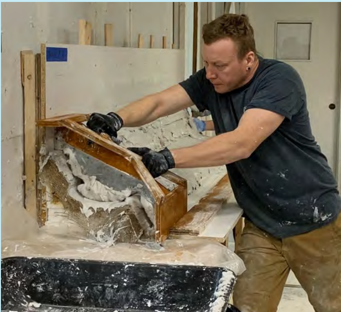
A plasterer pushing the slipper along the bench. This process is carried out about 40-50 times within a 20–25-minutes timespan.
