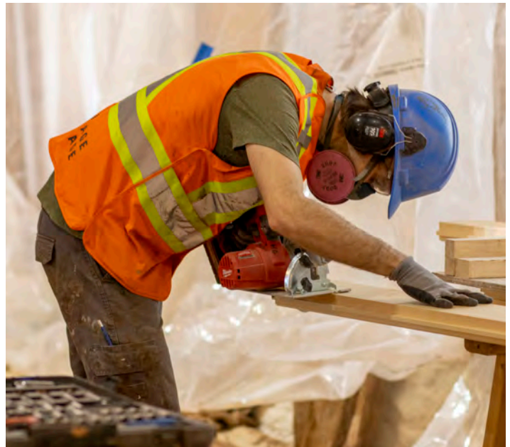
The carpentry team is replacing any worn or rotten pieces of the floors with white pine – the same material used originally.
