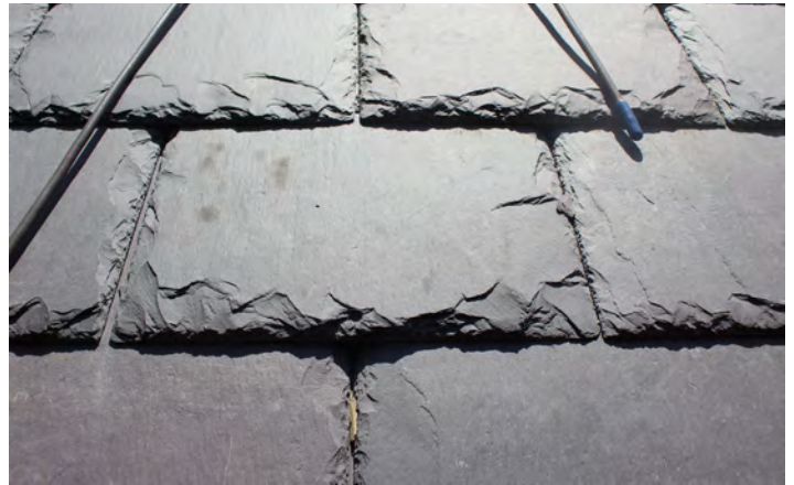
A close-up image of the new slate shingles at Province House National Historic Site. The new slate is sourced from the same location when Province House was constructed between 1843-1847.
