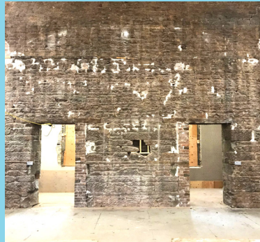
An image of the West Pavilion wall, located in the Confederation Chamber, before conservation work began.
