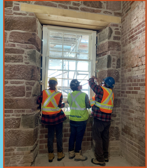
Students carrying out the intricate reinstallation process of these centuries old windows at Province House National Historic Site.
