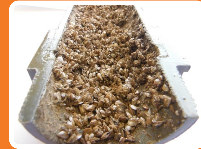
Water intake pipe clogged with mussels. Photo: Province of Manitoba
